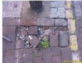
05 September 2007 More Details Available Block paving missing - trip hazard Highways outside 26 catbird bdy, rear town hall.
