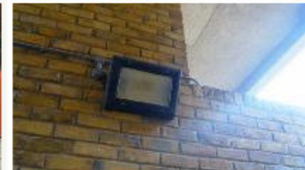
05 September 2007 PLEASE REPLACE DEFECTIVE LIGHT BY THE MAIN ENTRANCE OF LEYBOURNE HOUSE. REPORTED BY NEW/CROSS WARDEN
